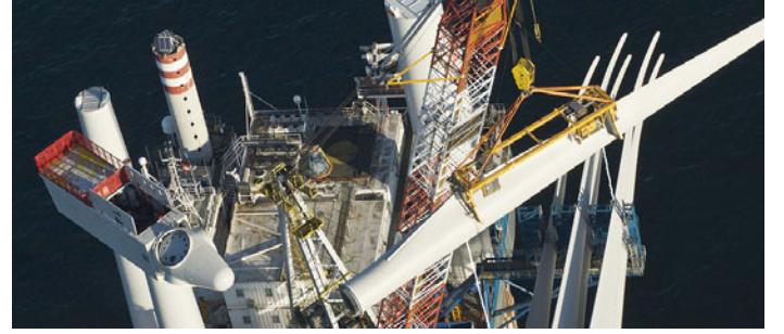
Fig. 1 Illustration of the mating phase during a single blade installation (image source: Schneider (2014)).
